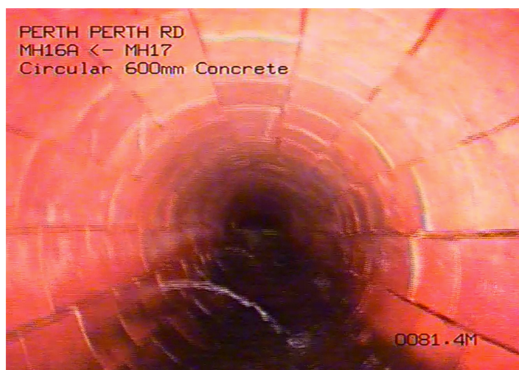
Figure 39. CCTV survey image of the barrel drain
