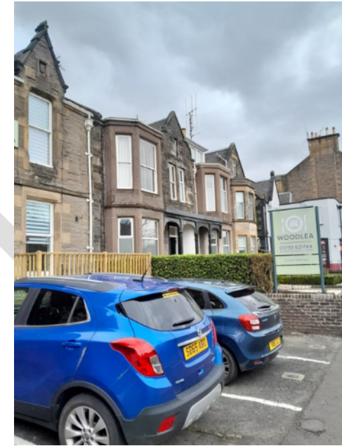
Figure 85 – Eroded front boundaries along York Place
