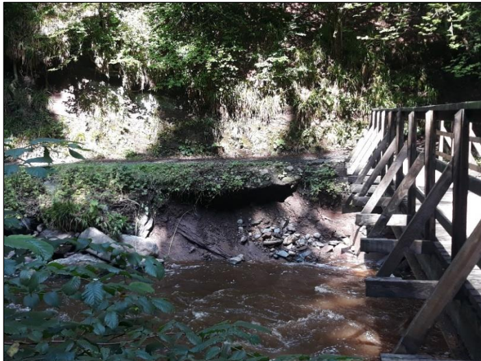
Photo: Path erosion
